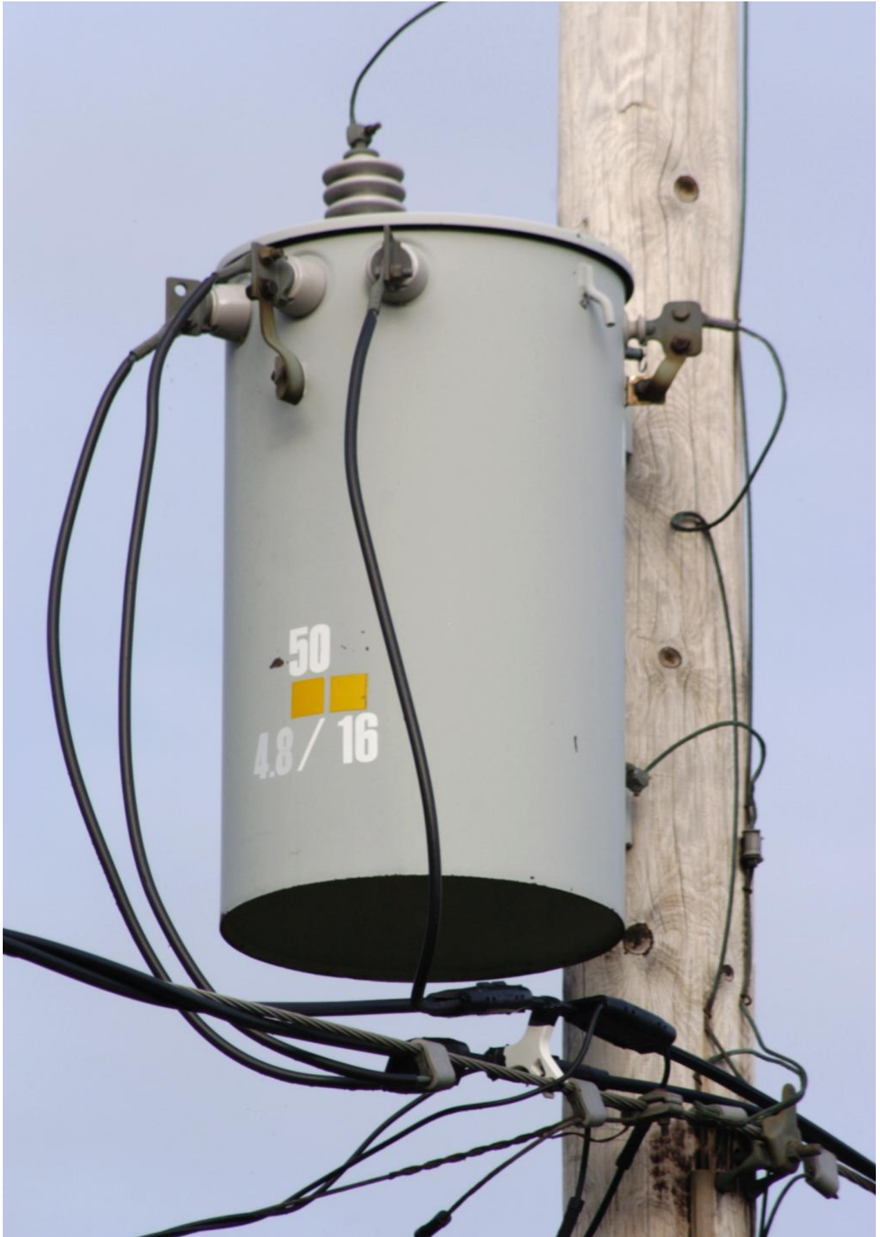
Small introduction to Transformer
